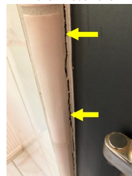
Deficient back wall seal
