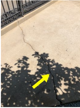
Right side patio cracking
