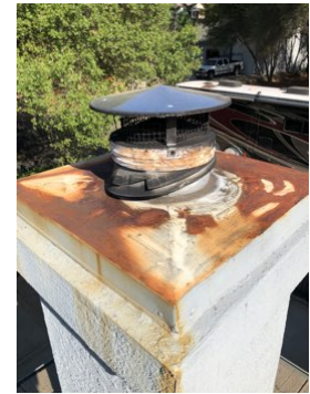
Rusted metal chimney crown
