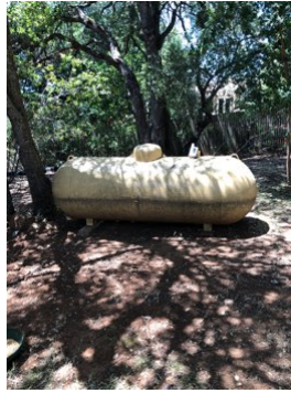
Liquid propane tank detail
