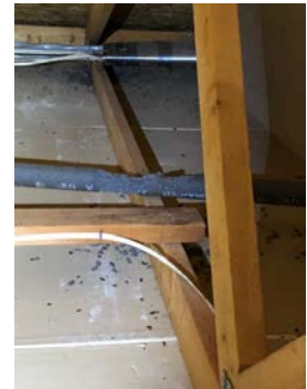
Pipe insulation rodent damage
