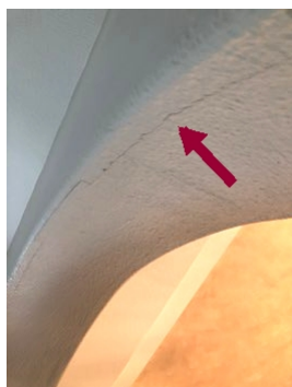
Dining archway cracking
