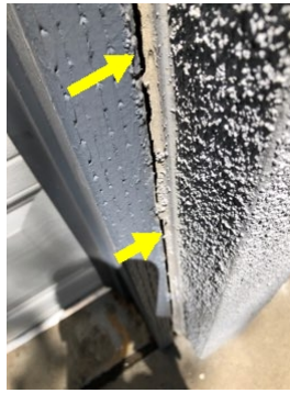
Deficient left vehicle door seal
