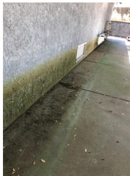
Rear stucco staining
