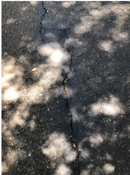
Asphalt driveway cracking
