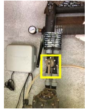
Water shut-off valve
