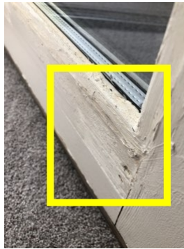
Door frame damage
