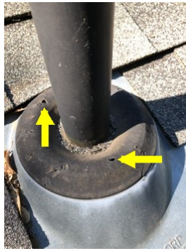
Holes in vent pipe rubber boot
