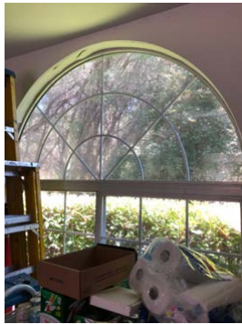
Possible failed seal
