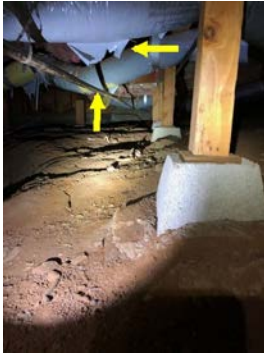
Torn duct pipe vapor barrier
