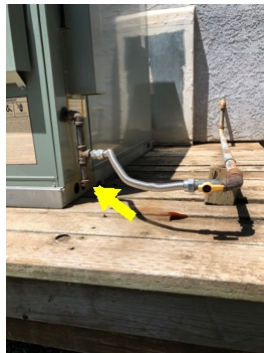
Gas line with sediment trap
