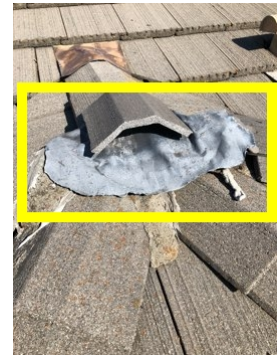
Questionable right ridge junction repair
