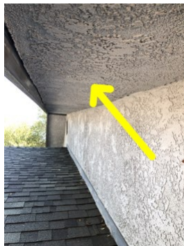
Sag in eave stucco
