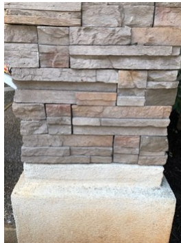
Drain plane not evident on columns
