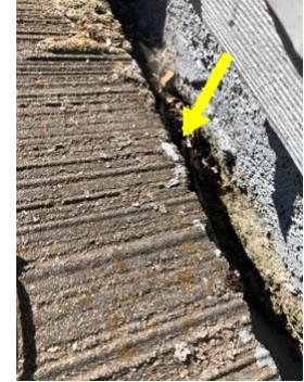
Clogged chimney 2 upper flashing
