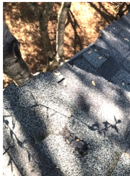
Right side tree branch roof damage
