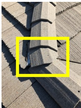
Loose rear right hip tile
