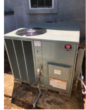
HVAC heating & cooling unit detail
