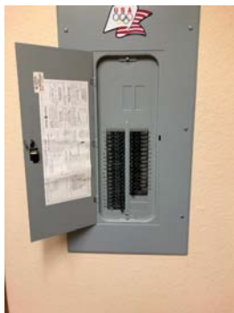
Main service panel detail
