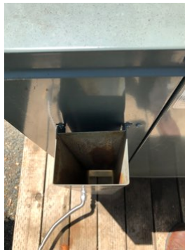
Missing exterior vent screen
