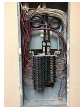
Main service panel detail
