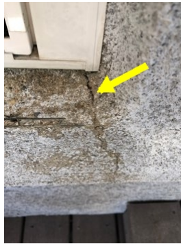
Rear right window trim cracking
