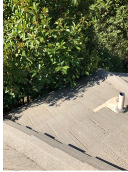
Tree branches overhanging roof deck
