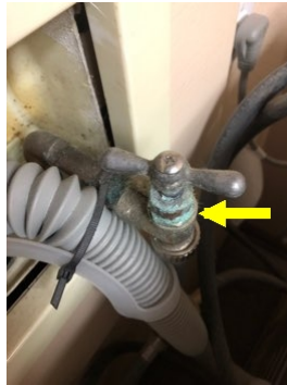
Corrosion on washer water valve
