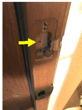
Missing strike plate
