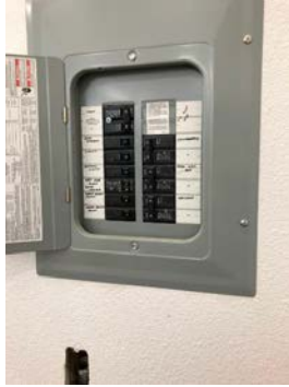
Detached garage sub panel detail
