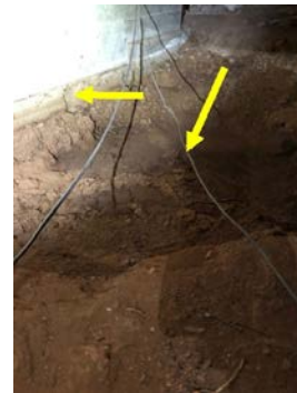
Large pit/exposed footing crack rear right
