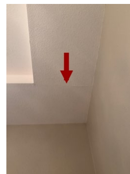
Dining room ceiling seam
