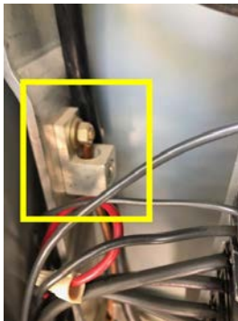
Grounding electrode wire panel attachment
