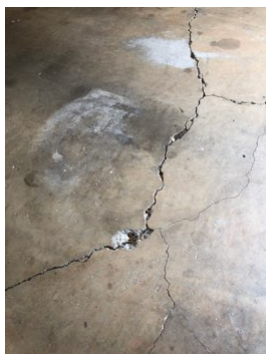
Significant concrete floor cracking
