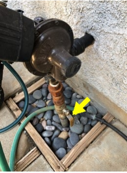
Secondary gas shut-off valve
