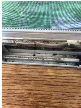
Cracked window screen seal
