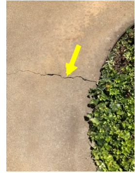
Rear patio cracking
