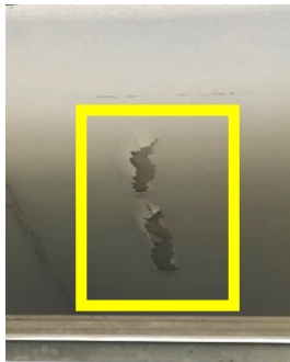
Peeling ceiling paint
