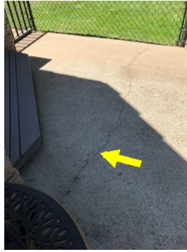
Right side patio cracking
