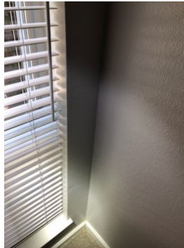
Wall corner patch
