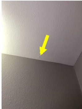
Ceiling nail pop
