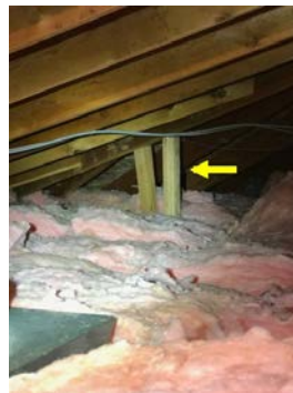
Questionable rafter support close-up
