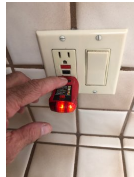
Deficient counter GFCI outlet
