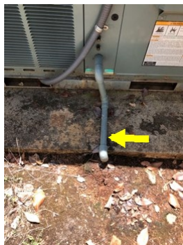
Missing trap on condensate drain line
