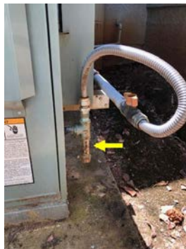
Gas line with sediment trap
