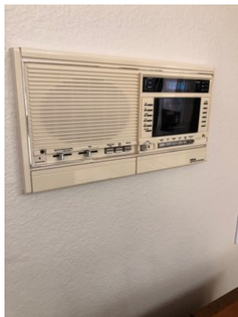
Intercom system control panel
