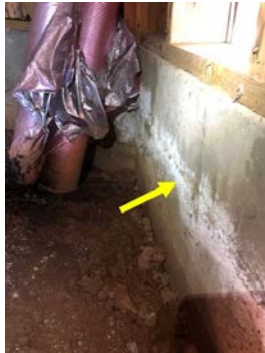
Efflorescence on foundation wall
