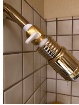
Leaking bath 3 shower head
