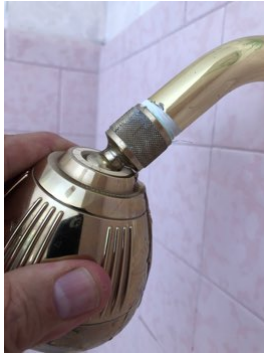
Leaking bath 2 shower head
