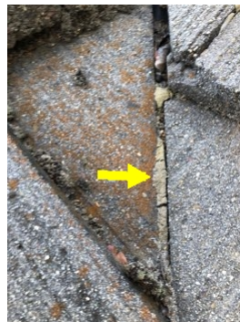
Moss clogging valley flashing
