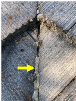
Moss clogging valley flashing
