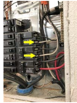
Unmarked white wire on sub panel
