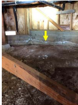
Efflorescence on foundation wall
