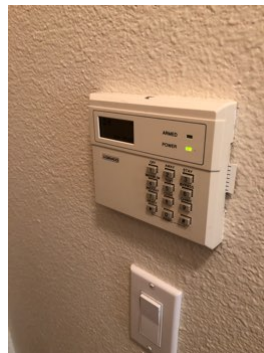
Security system control pad detail
