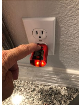
No half bath outlet GFCI protection
