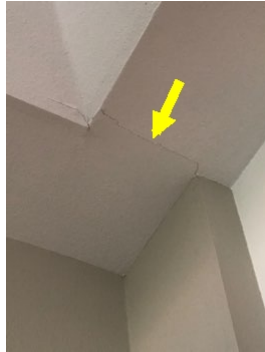
Living room ceiling crack
