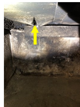
Broken firebox brick
