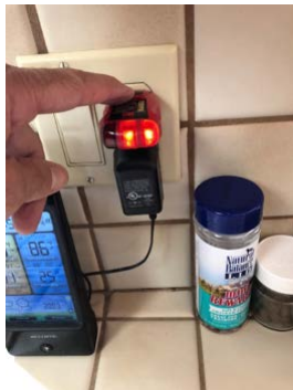
Deficient counter GFCI outlet
