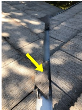
Loose tile on front center
