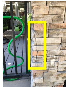
Deck railing stone column cracking
