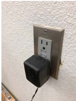
Right GFCI protected outlet
