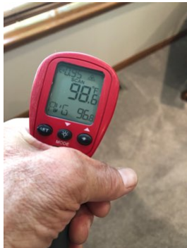
Master bedroom heat system register temp
