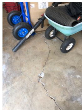
Significant concrete floor cracking
