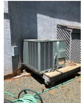
HVAC heating & cooling unit detail
