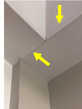
Living room ceiling crack
