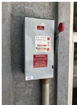
Main disconnect possibly for generator use
