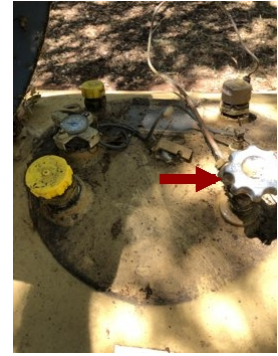
Liquid propane tank shut-off valve detail
