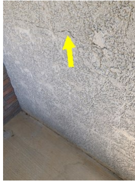
Rear stucco cracking
