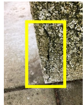
Rear stucco corner crack
