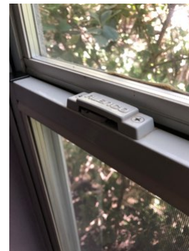
Broken bedroom 3 window latch
