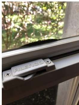
Broken bedroom 3 window latch
