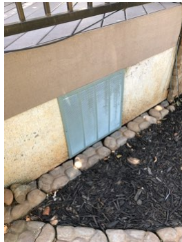
No access under deck
