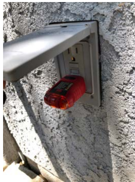
Deficient front right GFCI outlet
