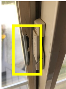
Damaged bedroom 4 exterior door
