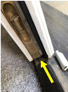
Living room inactive door would not open
