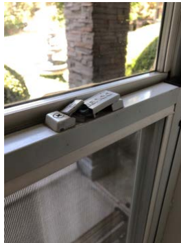
Living room window broken latch
