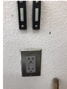
Left GFCI protected outlet
