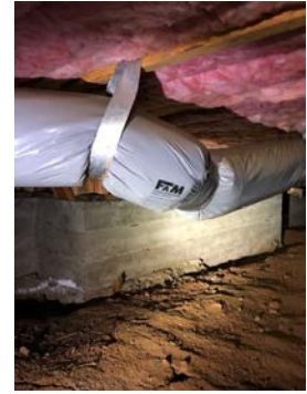
Restrictive duct pipe strapping
