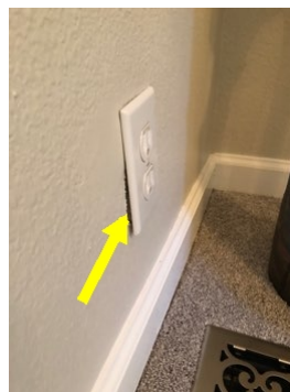
Dining room outlet not flush to wall
