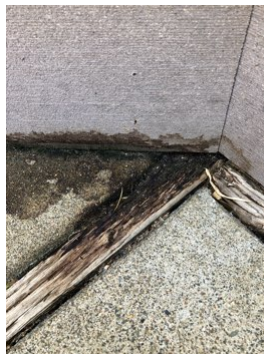
Right side landing moisture damage
