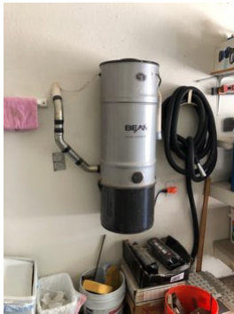
Central vacuum cleaner unit detail
