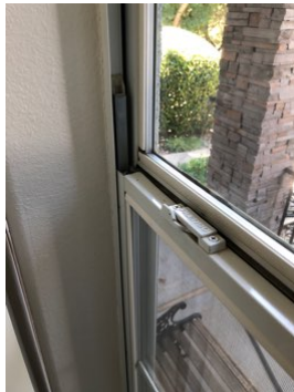
Living room window broken balance spring
