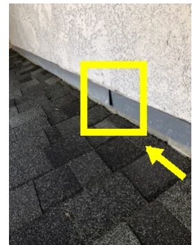
Wrong overlap on stucco sidewall flashing
