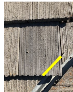
New tile not cut for valley flashing
