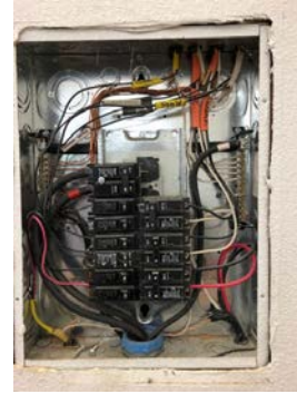
Detached garage sub panel detail
