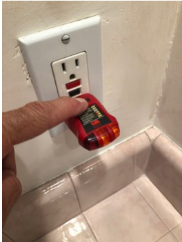
Deficient bath 2 GFCI with power on
