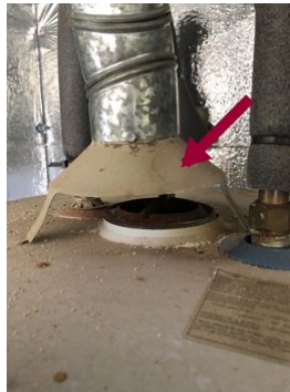
Misaligned vent pipe
