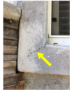
Window trim cracking
