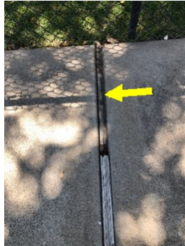
Wood decay on right patio expansion joint
