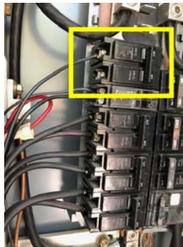
Half loaded 2-pole breaker in main breaker box
