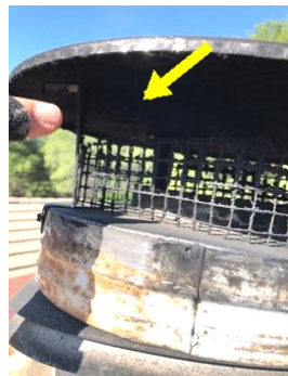
Large gap in spark arrestor
