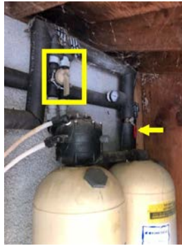
Water shut-off valves
