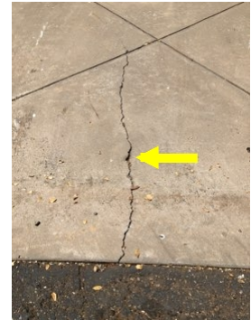
Detached garage driveway cracking
