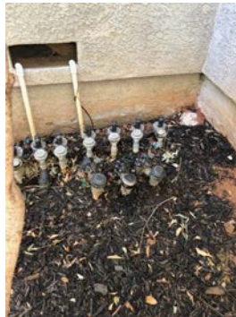
Irrigation system sprinkler valves
