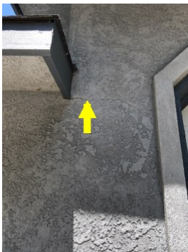
Front stucco crack
