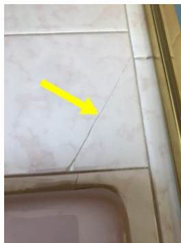
Cracked tub deck tile
