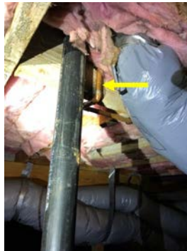
Missing copper pipe insulation
