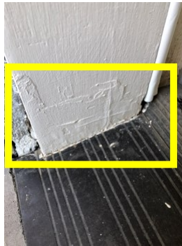
Patched door jamb bottom
