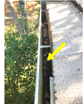
Gutter clogged with organic material
