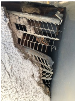
Exposed eave stucco lath with no backing
