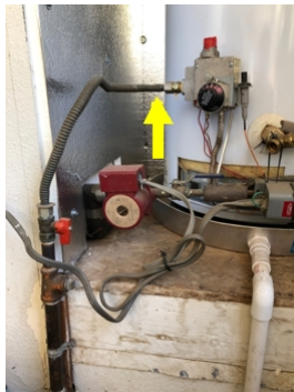
Gas line without sediment trap
