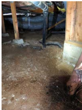
Damp crawlspace soil
