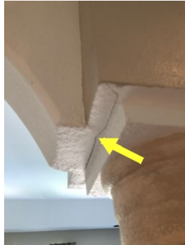
Left living room column crack
