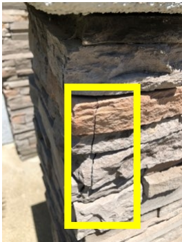
Deck railing stone column cracking
