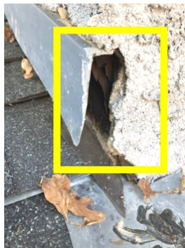
Front gap in flashing
