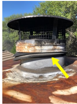
Loose chimney flue collar
