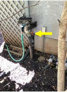
Secondary water shut-off valve
