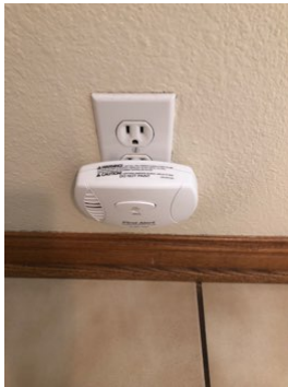
Hallway CO alarm detail
