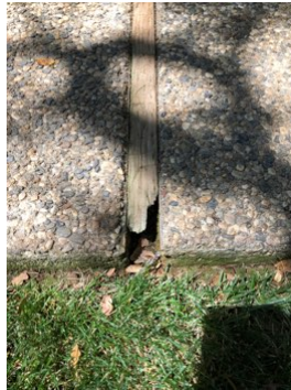
Front walkway expansion joint wood decay
