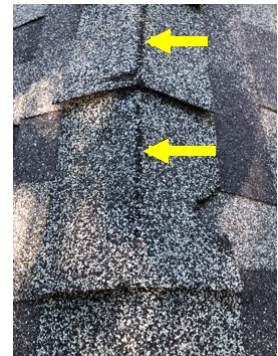
Ridge shingle splitting
