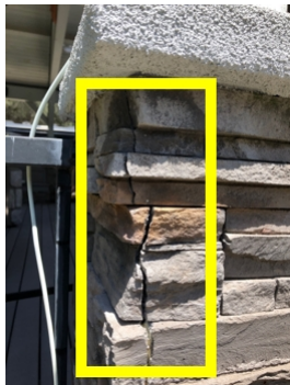
Deck railing stone column cracking
