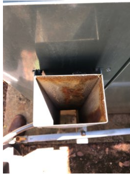
No exterior vent screen
