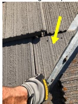
Loose valley tile
