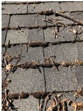
Moss on shingle roof
