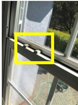
Broken latch in toilet room
