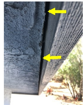
Stucco separation from barge rafter
