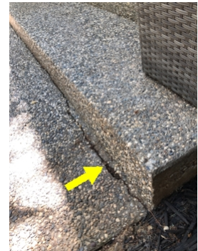
Concrete entry stair base cracking
