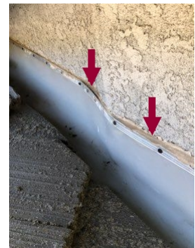
Questionable sidewall flashing
