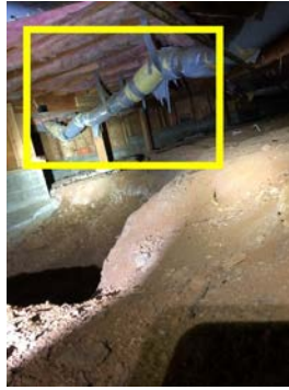
Torn duct pipe vapor barrier
