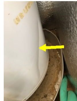
Outer shell damage
