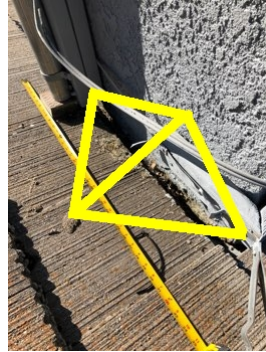
Missing cricket to divert water
