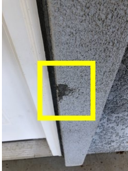
Left stucco trim damage
