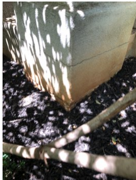
Left column bottom cracking
